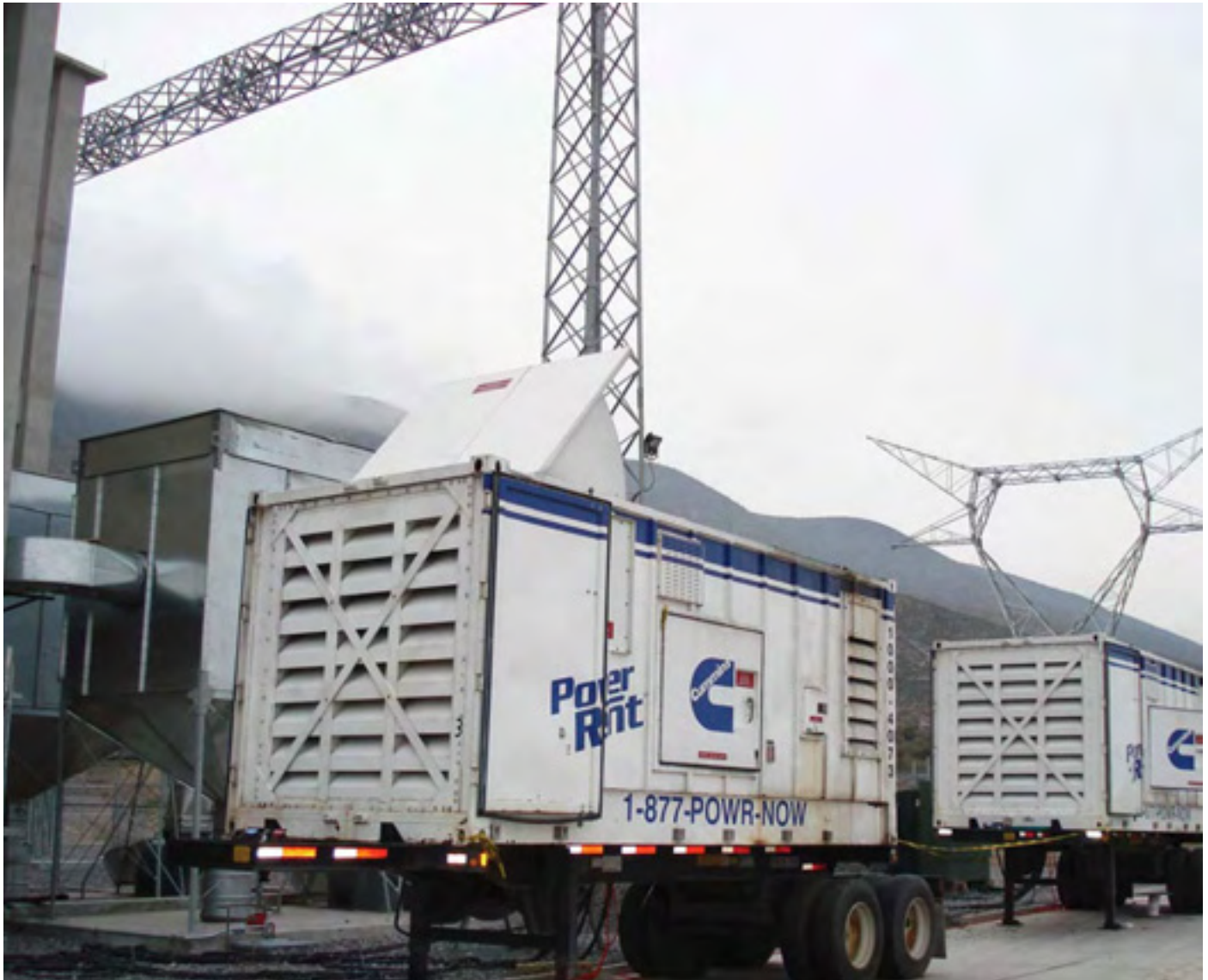
Thirteen Rental Power units from Cummins Power Generation power Cementos Cruz Azul while the large transmission line is completed.
