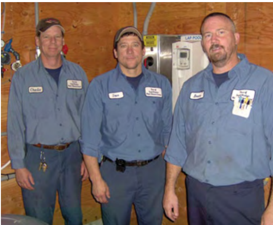
Charlie Albert, Dave Geng, and Bruce Lundie (left to right) handled the installation of all the ABB drives, operating the filtration pumps for the three pools in South Windsor, CT.
