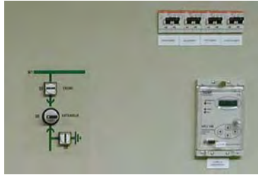
Figure 9. VAMP 140 relay installed at Rautaruukki.
