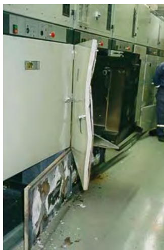
Figure 1: A cubicle damaged by arc short-circuit.
