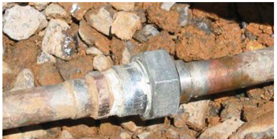
One type of dielectric coupler (union) installed in water line.
