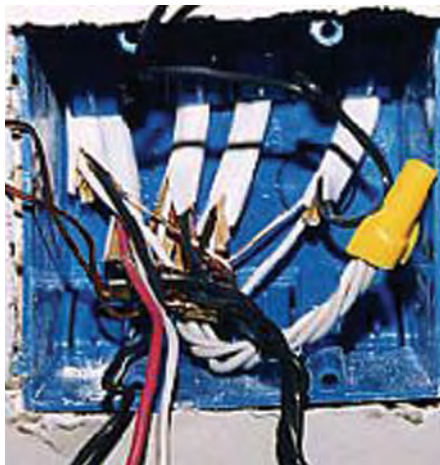
Electrical Wiring Box
