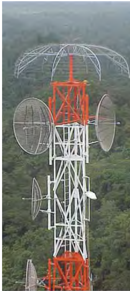
Dissipation array system mounted to a communications tower.
