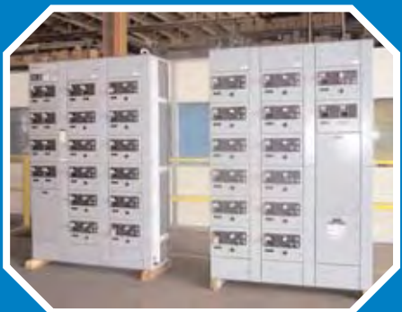
Motor Control Centers
