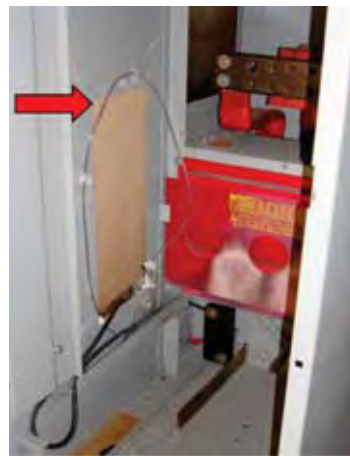
Fig. 6 Optical Fiber Sensor in the Breaker Compartment
