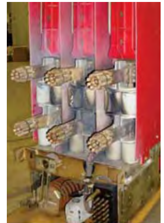
Fig. 7 Failed Westinghouse DHP Breaker
