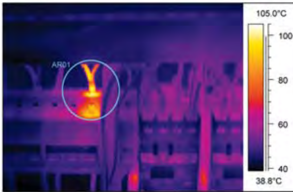
Distribution Board: Loose cable connection
