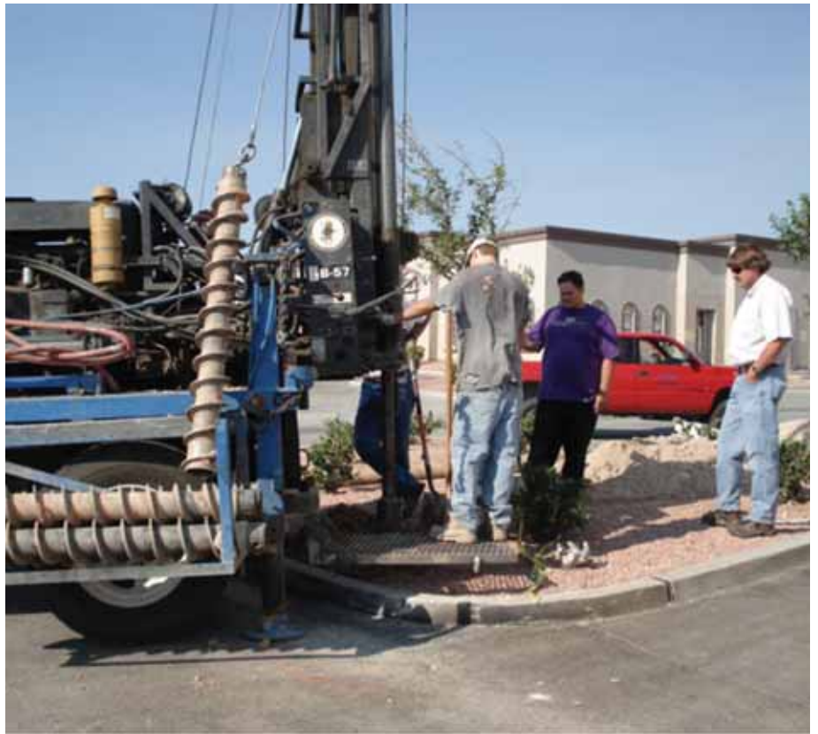
Typical installation involves trenching for the grounding conductors and in this case coring two 10 foot holes for installation of the XIT Grounding Systems.
