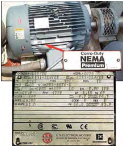
Figure 4. A 40-hp NEMA Premium-efficiency pump motor installed on a cooling tower at one of Emory University's centralized chillers. The motor bears the NEMA Premium label, signifying a nominal rated efficiency of 94.1%. Guaranteed efficiency is 93.0%.
