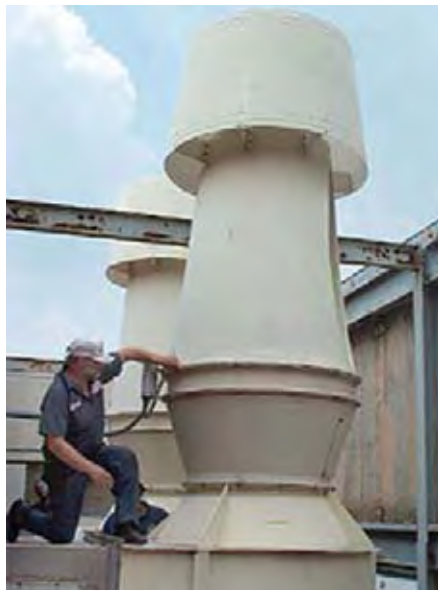
Figure 1. Two large exhaust fans on one of Emory University's research buildings. Emory design guidelines call for high-efficiency motors for its many chillers, air handlers, pumps and related equipment, which together account for more than 25% of the university's energy bill.
