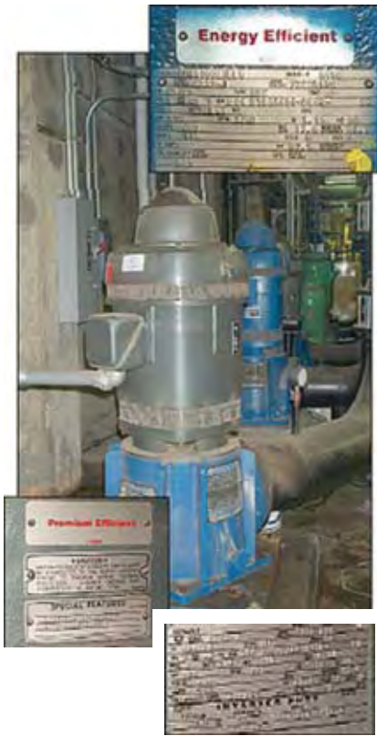
Figure 5. Three 100-hp cooling water pump motors serving an Emory University cooling system illustrate various commercial definitions for energy efficiency. The motor in the foreground has a nominal rated efficiency of 95.0% and carries a “Premium Efficient” label. 100-hp motors that qualify for the NEMA Premium rating have a nominal energy efficiency rating of 95.4%. Neither EPAct nor NEMA Premium requirements apply to vertical, inverter-duty motors such as the one pictured here. The blue motor (center) carries an “Energy Efficient” label and is rated at 94.1%. The average efficiency of older, standard-efficiency motors such as the green unit shown at the rear of the photo is 92.3%. To ensure a true “premium efficiency” motor, look for a NEMA Premium label, or compare the nameplate efficiency data to the NEMA Premium requirements.
