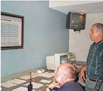
Figure 2: Each unit's efficiency loss, if any, is relayed to the system operator at a central control station and to Kicak's office PC as well as his PDA .
