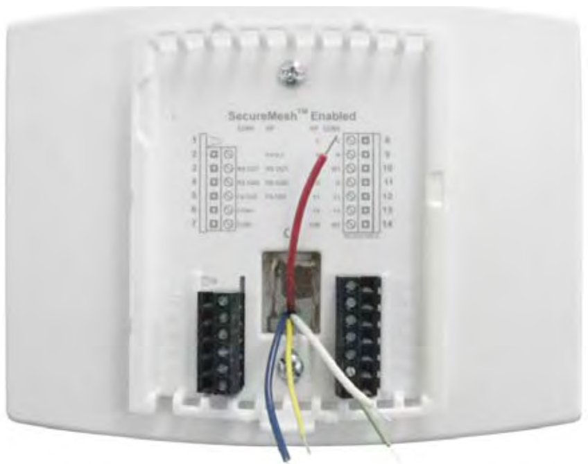
HVAC wiring colours and purposes vary - common wire may be missing.
